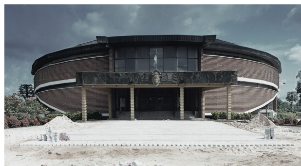
Figure 4. Exterior of the Oba Akenzua Cultural Center (during construction). Source: Authors’ fieldwork in 2019
