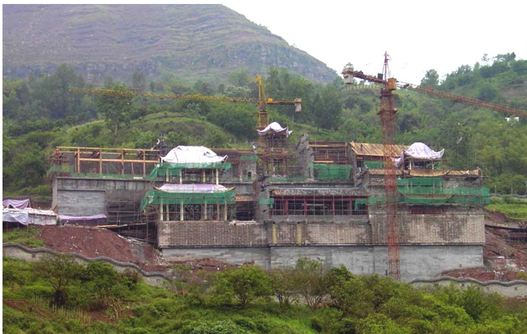
Figure 9. Restoration of Zhang Fei's Temple at the new site. Source: Photo by the author
