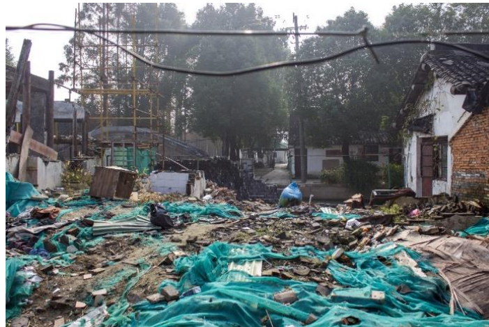
Figure 15. Unexpected demolitions found in Liantang. Source: Photo by Luca Maria Francesco Fabris, 2016
