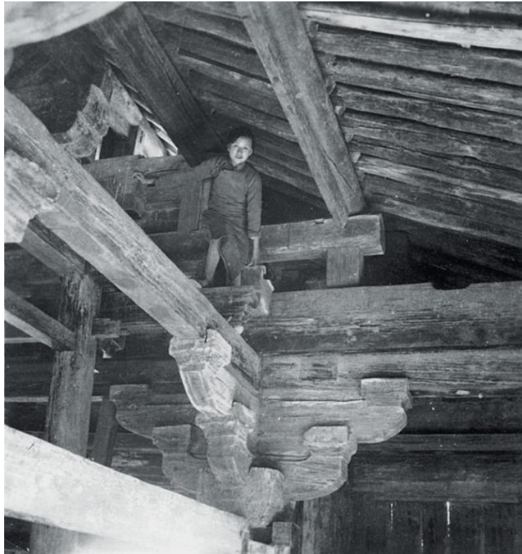
Lin Huiyin conducting a survey on the bell tower in the Kaiyuan Temple, Zhengding County, Shijiazhuang, Hebei Province, China (1933)
