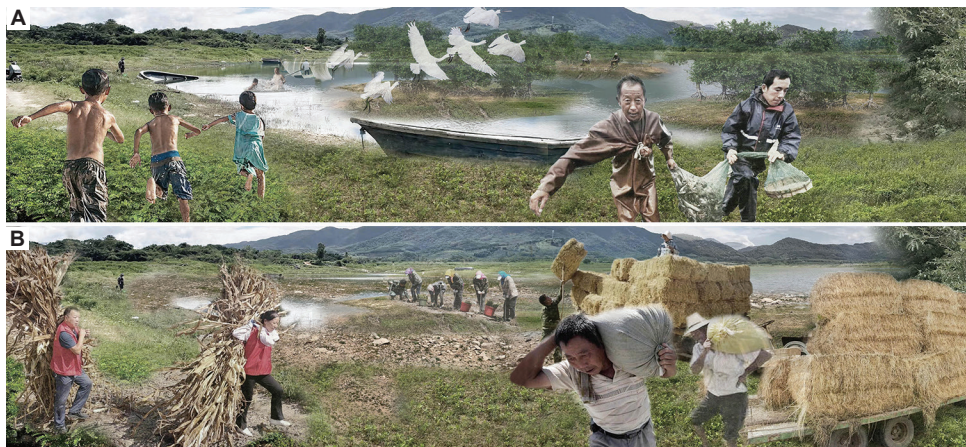
Figure 14. The participation of villagers in constructing the wetland area. (A) Rain season. (B) Dry season. Source: Photo combinations by the authors
