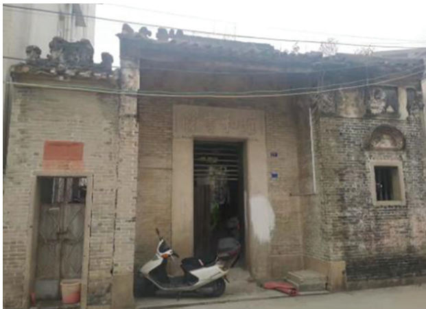
Figure 8. Damaged Yonghe Academy. Source: Photo by the authors
